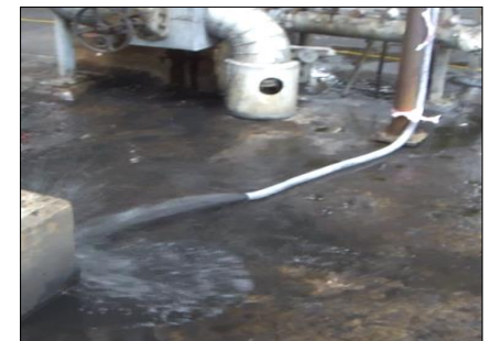
Waste water drain
