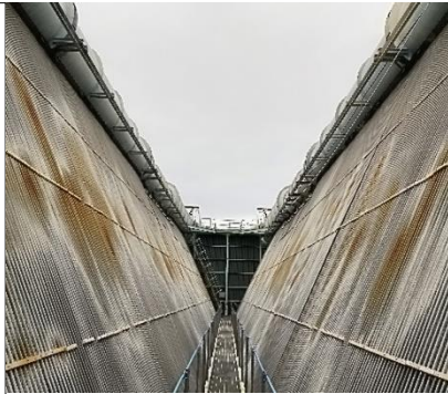
Air cooled condenser scales (Power Plant)
