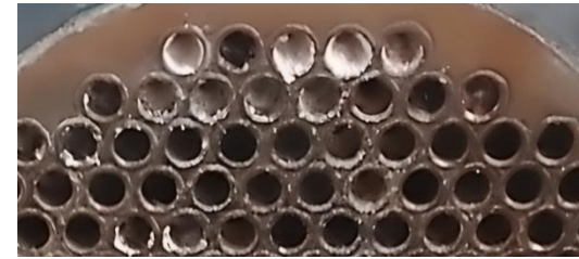
Cooling wafer tube side fouling
