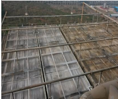
Air cooled condenser scales (Refinery)
