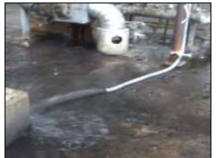
Waste water drain
