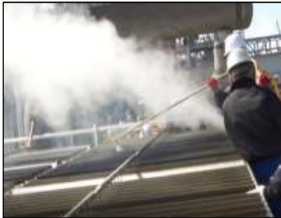
Top spray , online-cleaning
